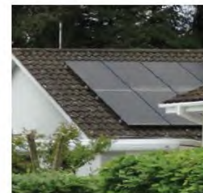
Roof solar panelling.
